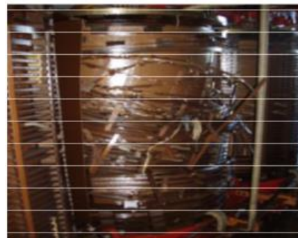
(a) Axial defects of HV winding with H2-H3 phase moved downward
