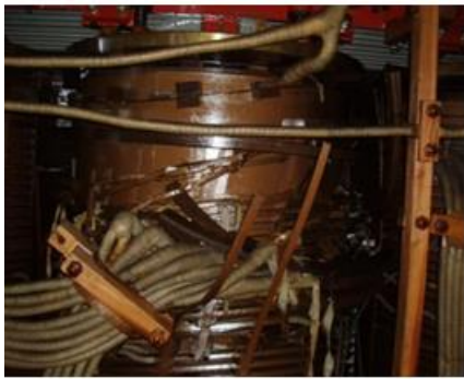
(b) Winding defects at H2-H3 phase affecting the tap leads winding
